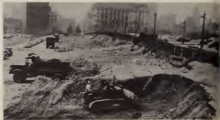
Excavation and grading of widened Adams Street, the new route to the Bridge.
